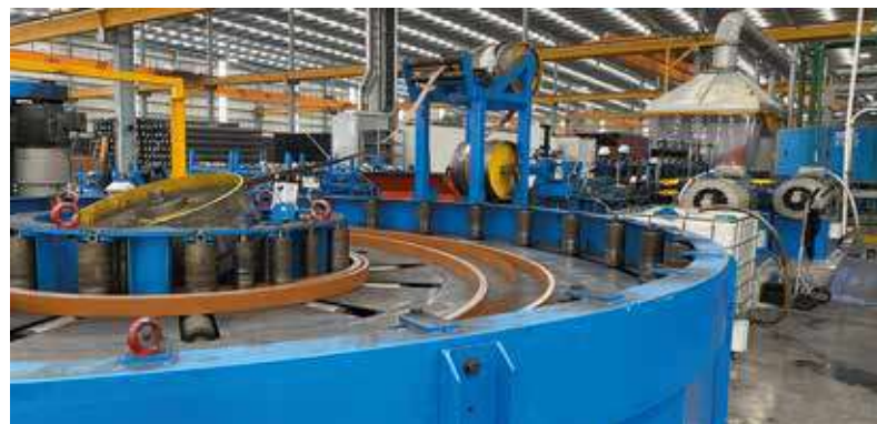
Pipe and RHS Plant
